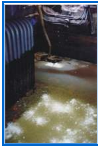
A sump pump is lowered through the solidified oil, lowering the water level from 3' to 6".
